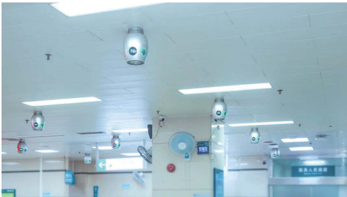
FIGURE 1. Ceiling oxygen equipment in the outpatient hall.
