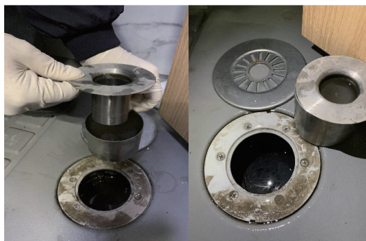
SUPPLEMENTARY FIGURE S5. The figure of the floor drains and removable water trap in a centralized quarantine apartment in Beijing.
